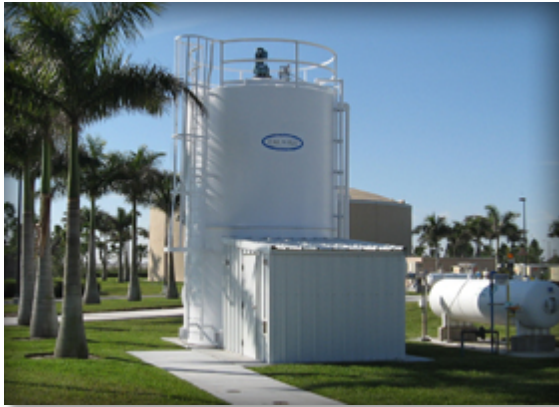
Figure 3 – Burnett Lime feed equipment for neutralization and
