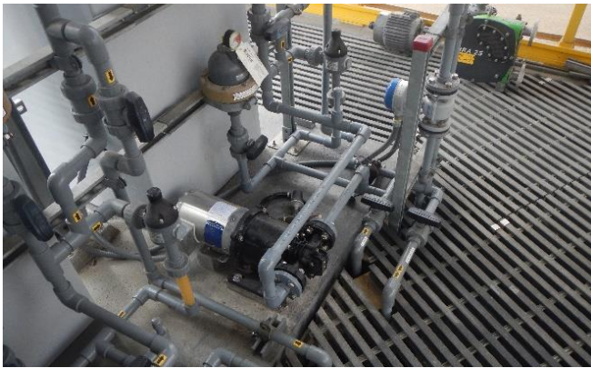
Figure 2 – The City of Escondido Water Treatment Plant replaced peristaltic pumps with Pulsafeeder Eclipse E25 and E125 Hypo Gear Pumps
